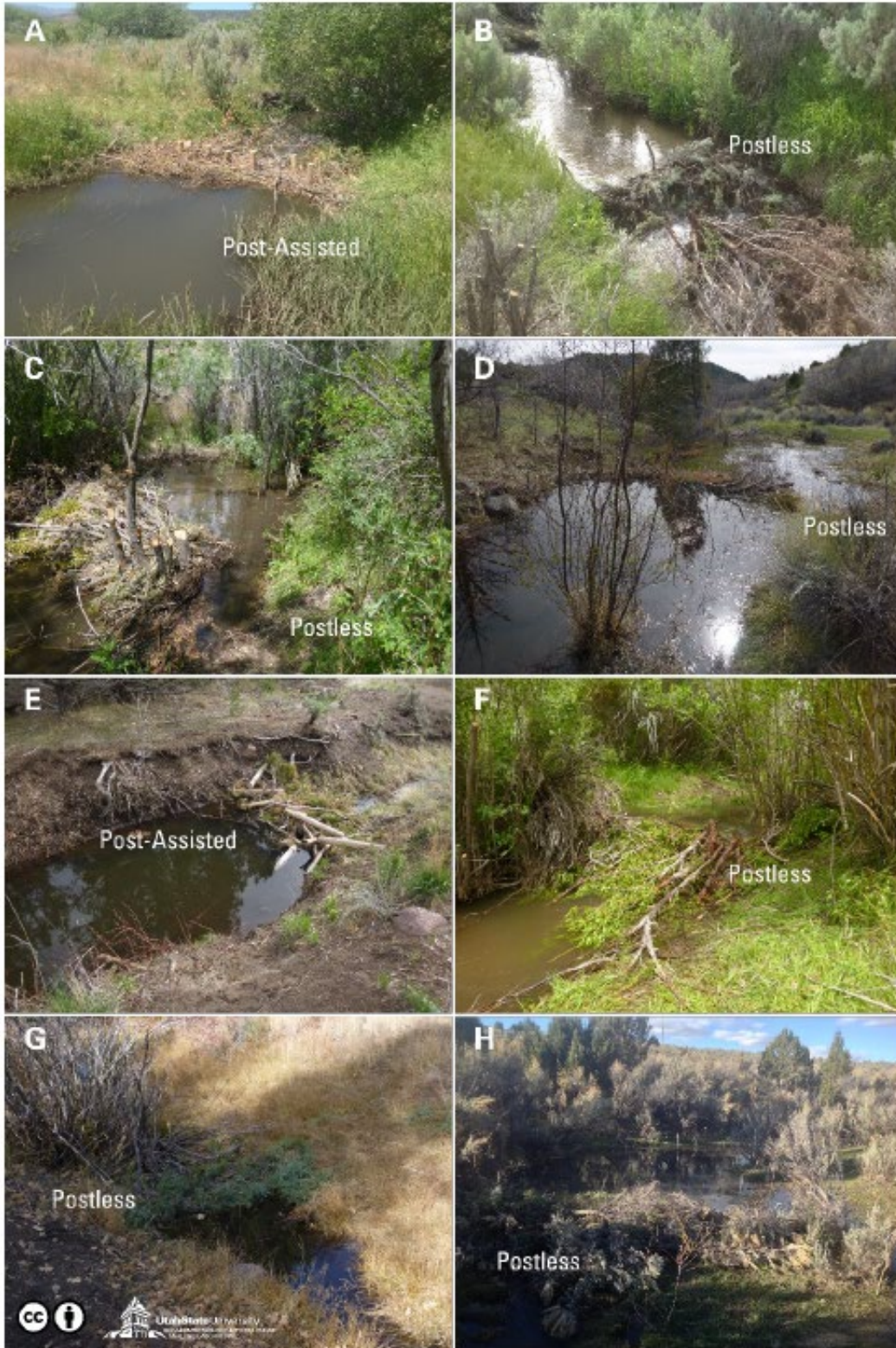
Figure 23. Examples of BDAs built in a range of settings, using a variety of materials, and with or without untreated wooden posts for additional temporary stability.
