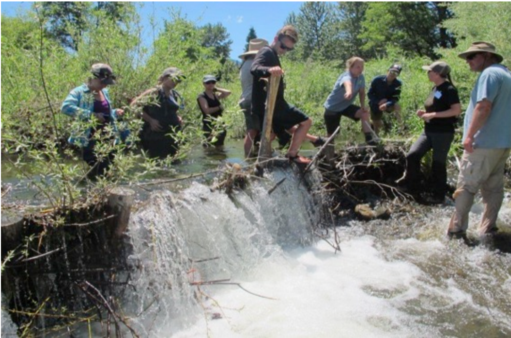
Photo Don Flickinger 6/2017. Sugar Creek BDA 0.1. Section of BDA that lost posts and was repaired with handtools evident by slightly lower profile and water spilling over the top.
